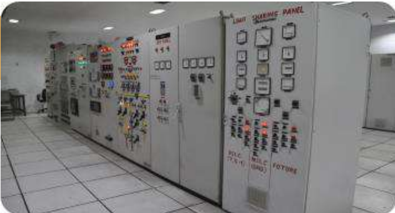
Cogeneration control panel
