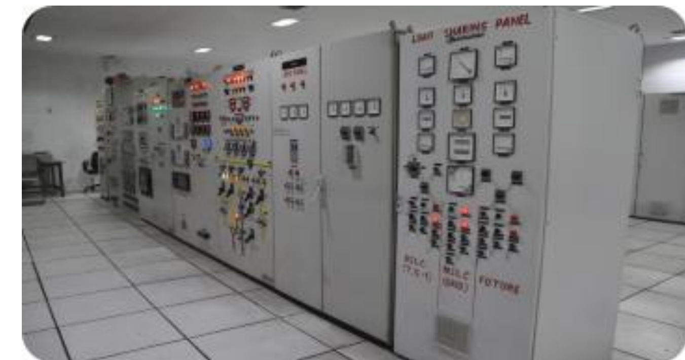
Cogeneration Control Panel
