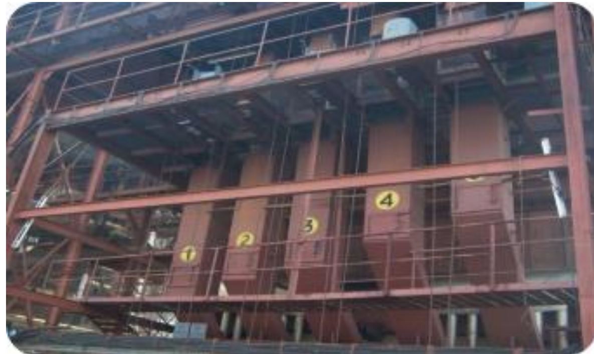
Bagasse Silos & Feeders of Boiler
